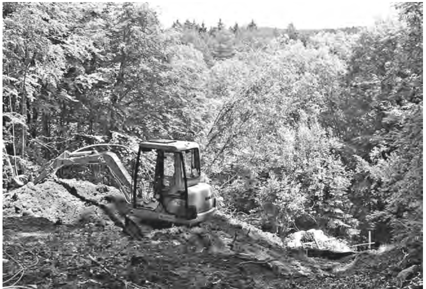
Figure 1. 2005 excavation showing machinery used in preparation of the Western Quarry. – Photographs: by the authors, if not noted differently.
